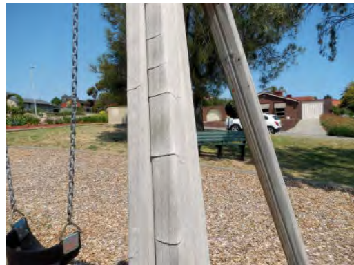
Photo taken: 28/11/2016 Swing frame exhibits cracking and splitting - monitor.
