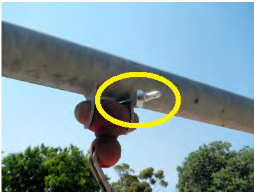
Photo taken: 28/11/2016 Pot'l finger trap due to height of swing frame.
