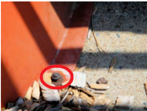
Photo taken: 28/11/2016 Exposed rusting fasteners.
