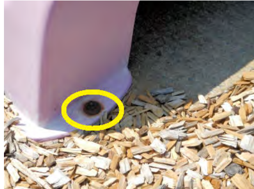
Photo taken: 28/11/2016 Exposed rusting fastener.
