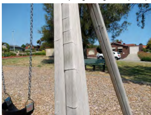
Photo taken: 28/11/2016 Swing frame exhibits cracking and splitting - monitor.
